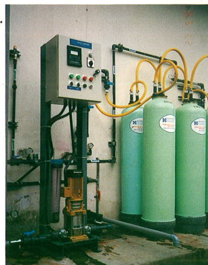
TWO BED COLUMNS
